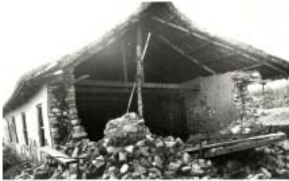
Figure 3: Typical failure of stone house during 1988 Earthquake of East Nepal
