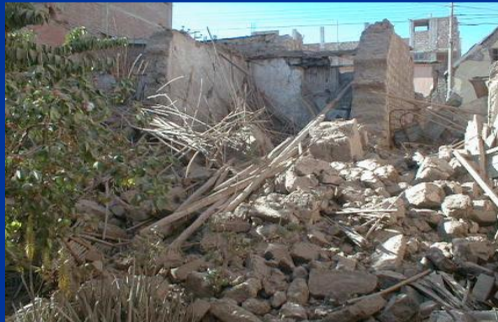
Damage to Adobe (2001 Atico, Peru EQ)
