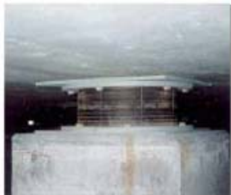
Figure 5.4.4 LRB on pedestal
