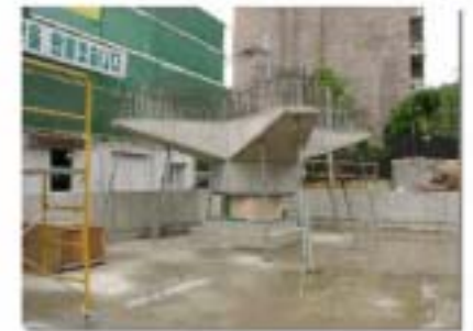
Figure 5.4.14 Load collector on a LRB
