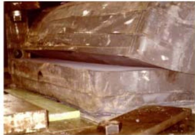
Fig. 5.23.d. Propagation of cracks between the layers of the bearing
