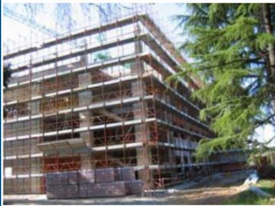
New isolated section of the Gervasutta Hospital using HDRBs
