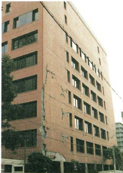
Photo . 3.2.1.65 Fracture of Anchor of Reinforcement
