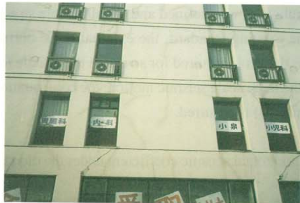
Photo. 3.2.1.42 Damage of beams mullion non-structural wall
