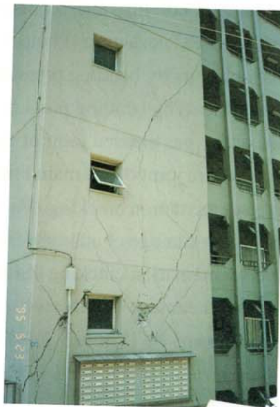
Photo. 3.2.1.15 Damage condition of the neighboring building (7 story frame structure; different one from the one of Photo. 3.2.1.14)
