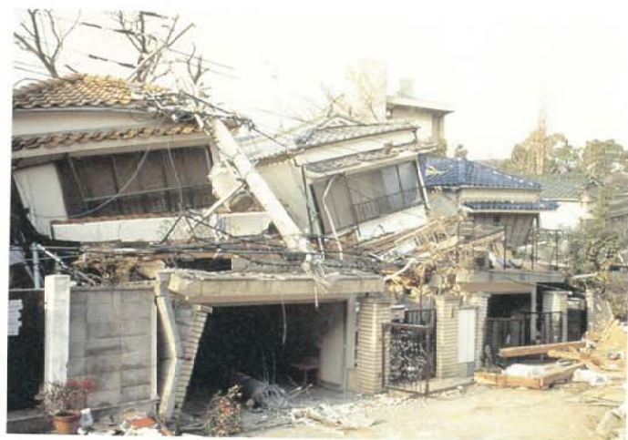
Photo 3.2.3.6 Collapse of the second story ( a garage of RC in the first story )
