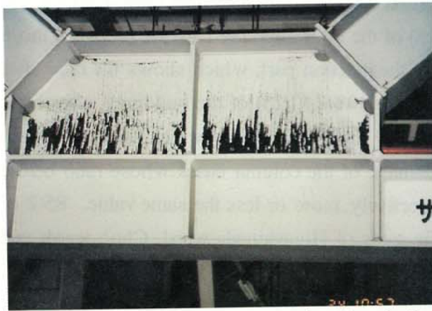
Photo 3.2.2.20 Shear yielding in the gusset plate at brace junction (Building C)
