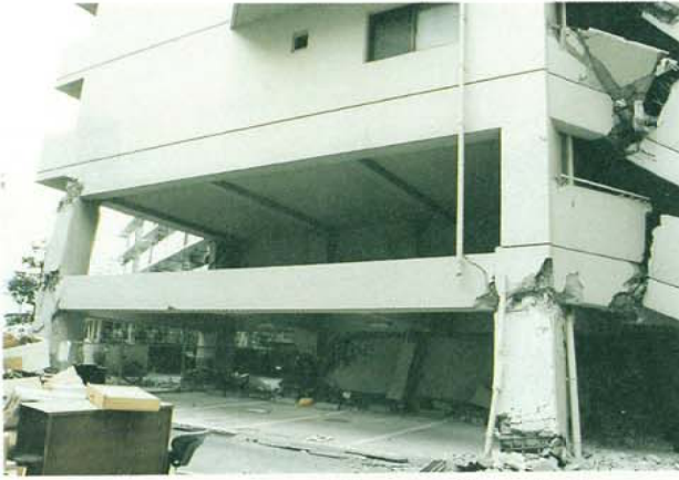
Photo. 3.2.1.33 Fracture of the top and base of columns
