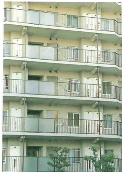
Photo . 3.2.1.66 Damage of Non-structural Partitions
