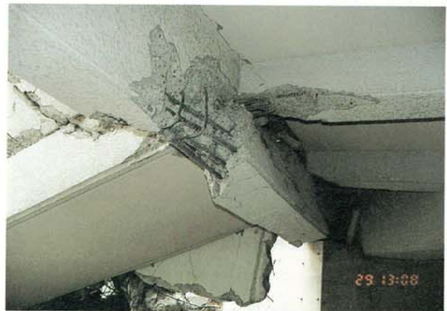
Photo. 3.2.1.32 Twist fracture of a beam
