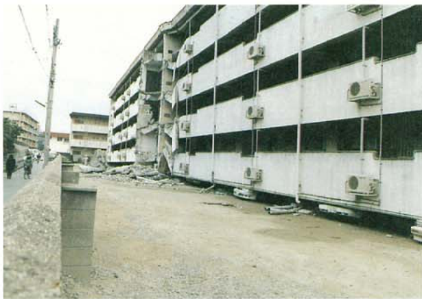
Photo. 3.2.1.2 5 story apartment house building Collapse of the first piloti floor
