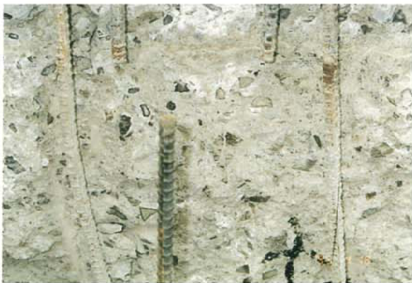
Photo.3.2.1.69 reaction rim around coarse aggregate by alkali aggregate reaction
