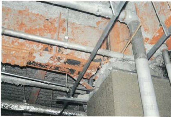
Photo 3.2.2.18 Fractured lower beam flange after largely plastic yielding (Building A)
