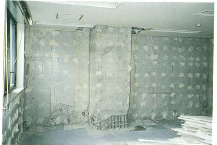
Photo. 3.2.1.36 Flexural compressive failure of columns
