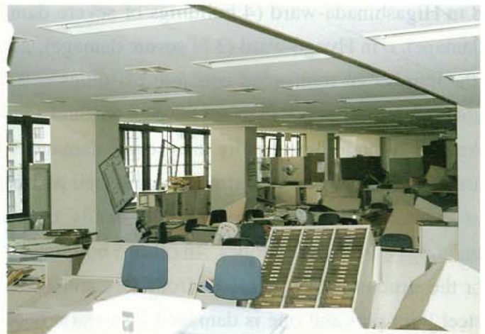
Photo. 3.2.1.48 Damage condition of the 7th roof floor of the 6th floor is pushed out to the 7th floor
