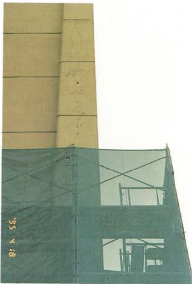
Photo.3.2.1.68 cracks along the axial direction Of column by alkali aggregate reaction
