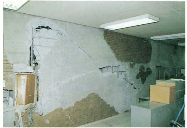
Photo. 3.2.1.4 3 story SRC structure governmental building The shear fracture of the yield strength wall (resistant wall) of the 7th floor
