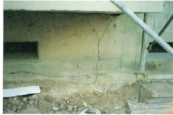
Photo. 3.2.1.13 Cracks of the base
