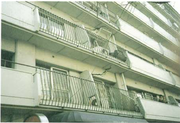
Photo. 3.2.1.41 Damage of beams mullion non-structural wall
