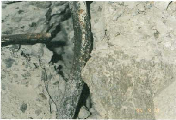
Photo.3.2.1.67 damaged hook by corrosion
