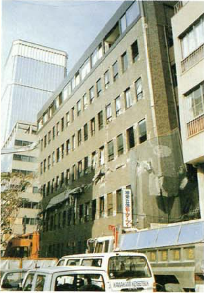
Photo . 3.2.1.58 Damage of 7 story Office Building
