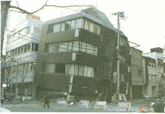
Photo. 3.2.1.1 4 story building Collapse by the shear fracture of the corner column of the first floor The story collapse of the piloti of the first floor
