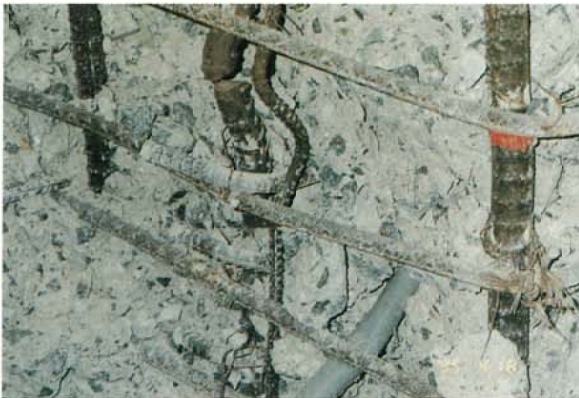
Photo.3.2.1.75 damaged gas pressure welded parts and not damage ones
