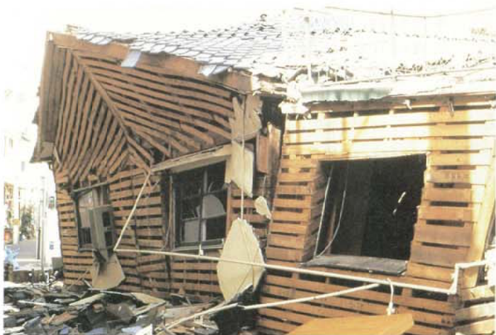
Photo 3.2.3.3 Collapse of the first story
