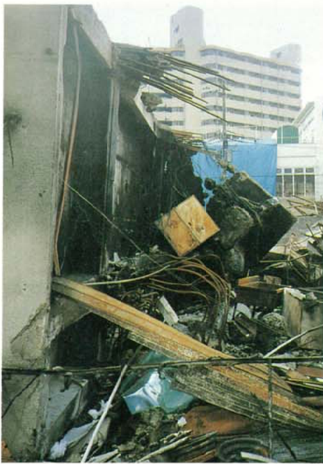
Photo. 3.2.1.18 Overturning of the whole building
