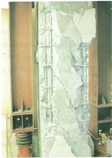
Photo. 3.2.1.39 Bond splitting failure of a column
