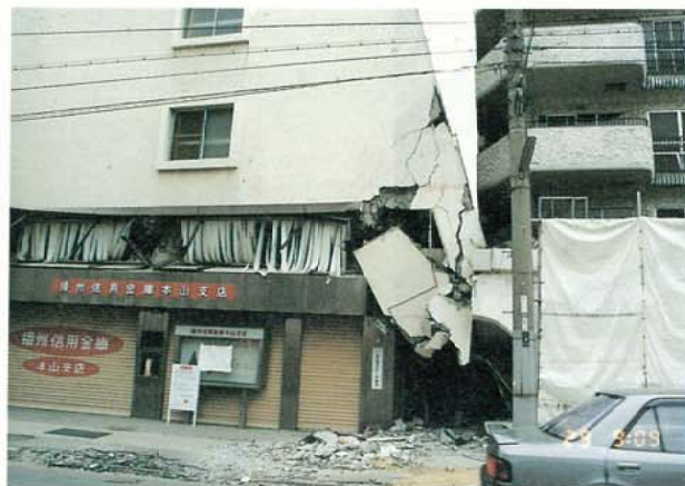
Photo. 3.2.1.26 Collapse caused by the collision of the buildings
