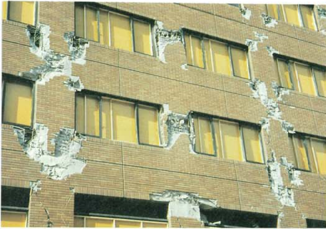
Photo. 3.2.1.35 Shear fracture Beam-column joints(SRC)
