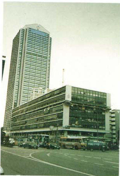
Photo. 3.2.1.3 8 story office building The 6th floor was suffered form the story collapse.(the building behind is non damaged)
