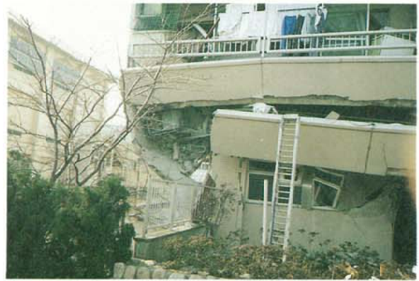
Photo. 3.2.1.5 7 story RC structured apartment house The story collapse of the second floor The number of the wall of the first floor is more than that on the upper floor. The shear fracture is seen on the column and the wall of the first floor.
