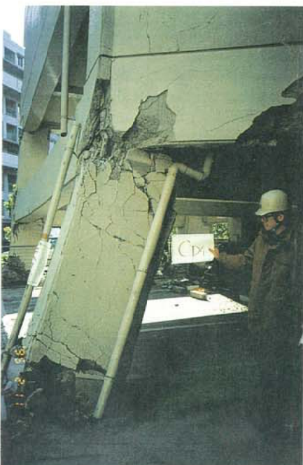
Photo. 3.2.1.53 Flexural Fracture (1FL)
