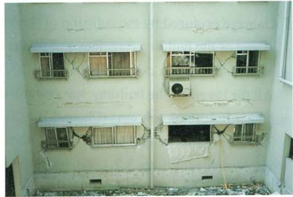
Photo. 3.2.1.14 Damage condition of the neighboring building (7 story frame structure)
