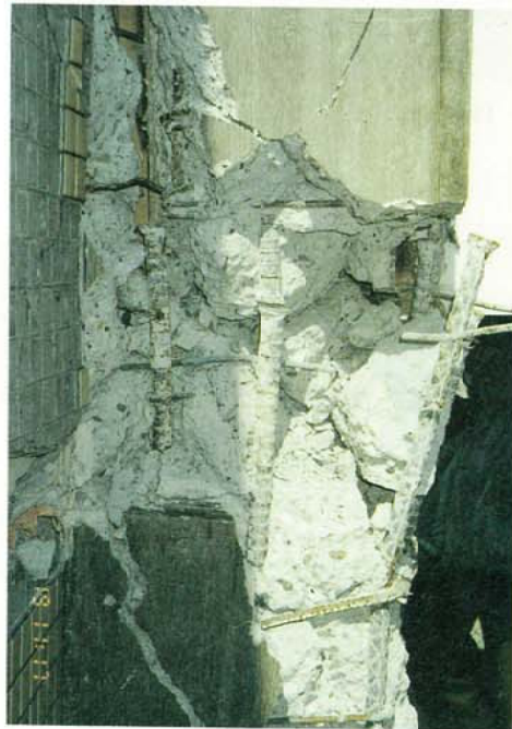
Photo.3.2.1.38 Fracture of the gas pressure welding of the reinforcements
