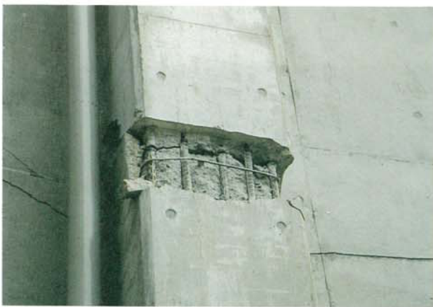
Photo. 3.2.1.37 Fracture of the gas pressure welding of the reinforcements
