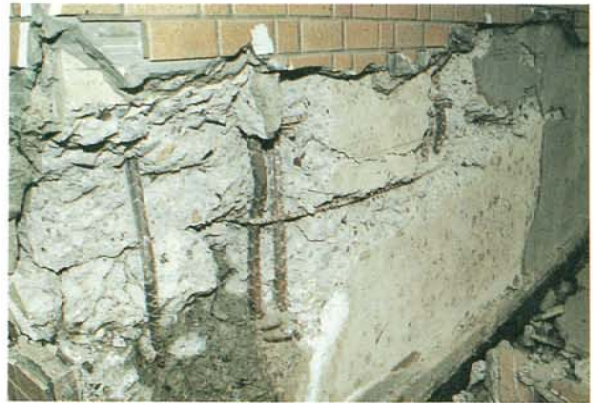
Photo . 3.2.1.64 Fracture of Splices of Steel
