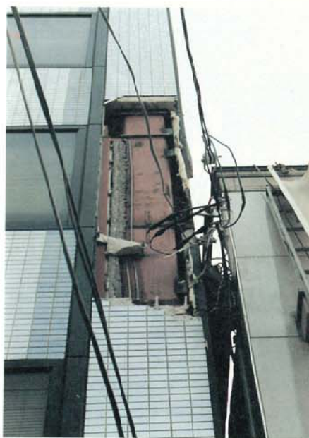
Photo 3.2.2.17 Two buildings collided.
