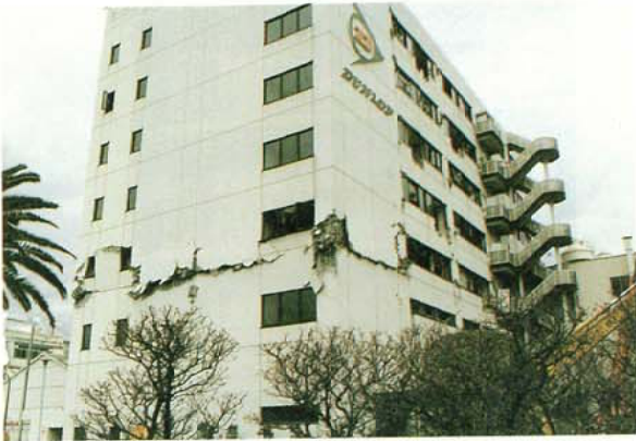
Photo . 3.2.1.60 Damage of relatively New Office Building
