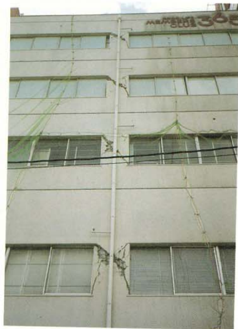
Photo. 3.2.1.30 Shear fractures of short columns
