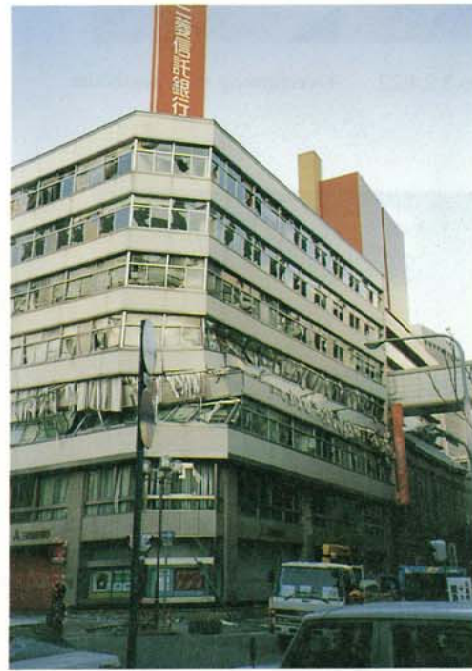
Photo. 3.2.1.19 Story collapse caused by the twist response
