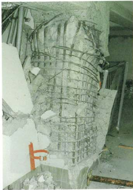
Photo. 3.2.1.55 Shear Fracture of Column(1FL,CD3) Rupture of Gas Pressure Welding of Longitudinal Bars
