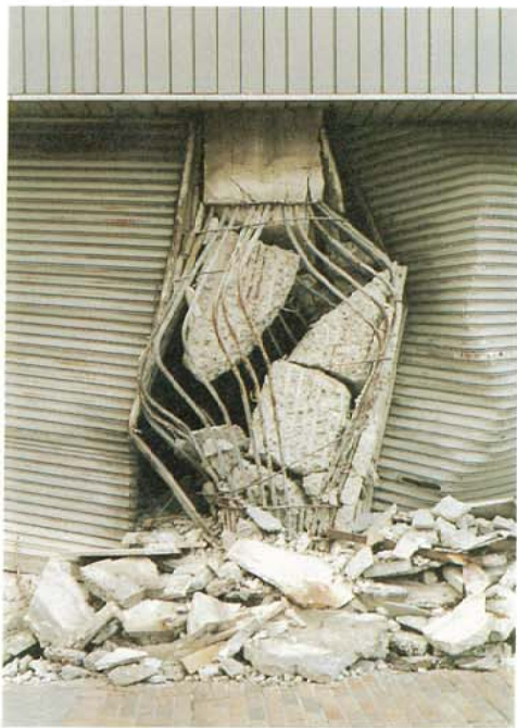
Photo. 3.2.1.29 Shear fracture of a column
