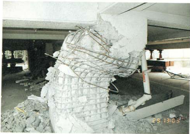
Photo. 3.2.1.31 Shear fracture of a column
