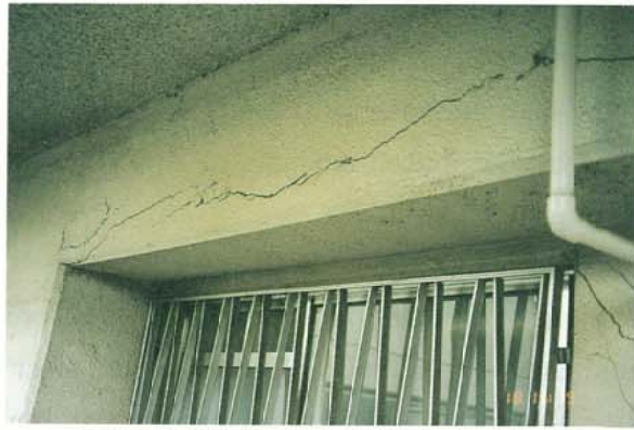
Photo.3.2.1.40 Bond splitting failure of a beam
