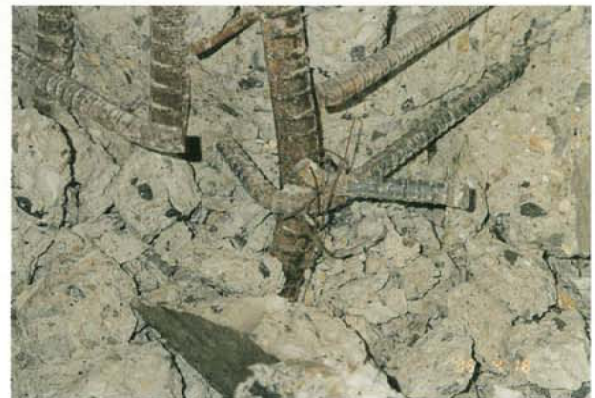
Photo.3.2.1.71 damaged bent part in reinforcement end
