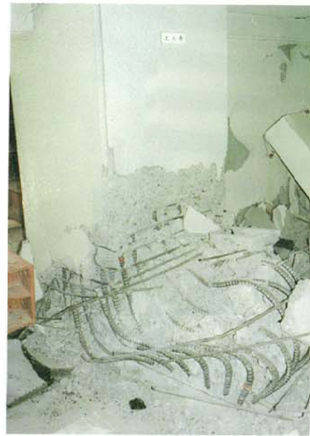
Photo. 3.2.1.56 Shear Crush of Column (1FL)
