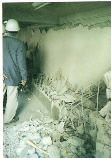
Photo. 3.2.1.54 Fracture of Shear Wall
