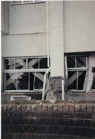
Photo. 3.2.1.8 4 story SRC structured office building The half of the column at the bottom of the anchor plate of the base of column was slipped to the north.
