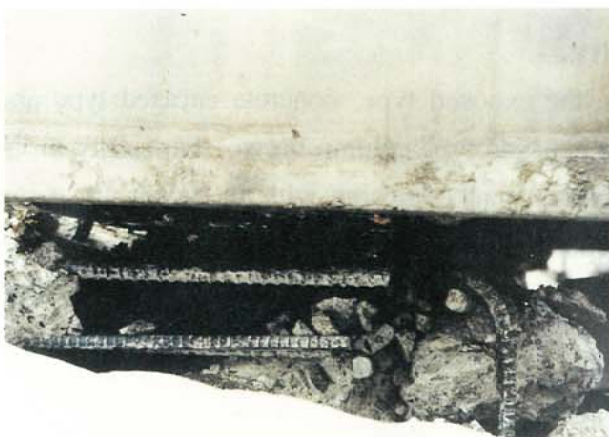
Photo 3.2.2.22 Damage of exposed column base (Building H)
