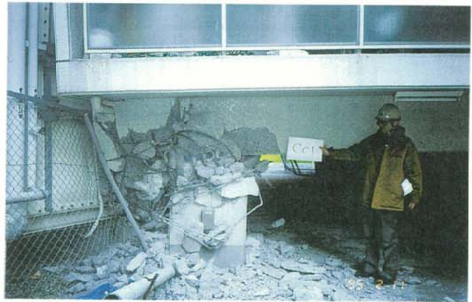
Photo. 3.2.1.52 Shear Fracture of 1 FL Column
