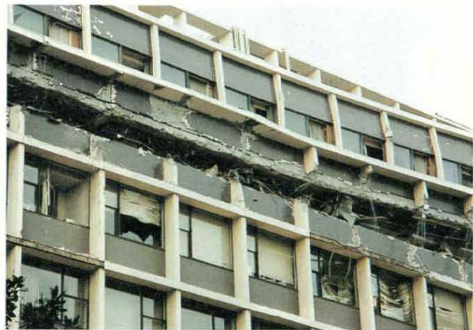
Photo. 3.2.1.25 Story collapse influenced by a set back
