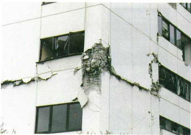
Photo.3.2.1.20 Fracture between the different structural types (SRC and RC)
