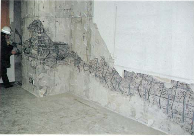
Photo. 3.2.1.7 11 story SRC structured governmental building Damage of the steel joint part of the peripheral column
